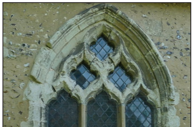
The stonework on many of the aisle windows is also badly eroded.
