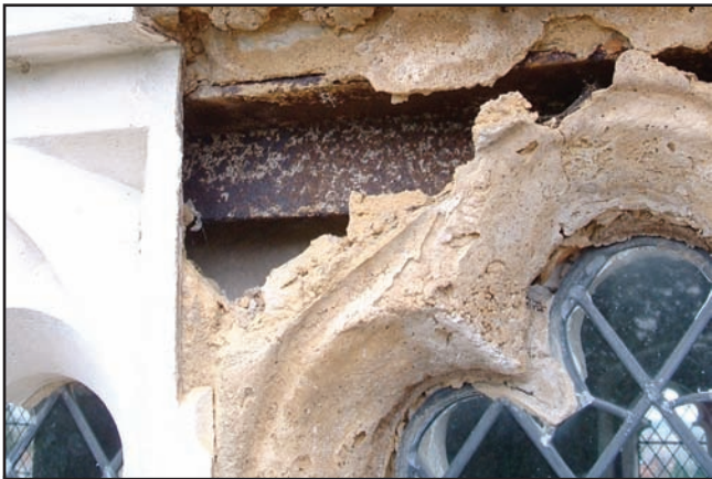
A close-up of a clerestory window on the South side showing behind the glass reinforced plastic facade.
